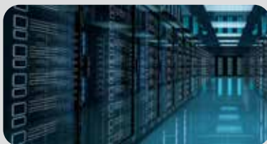
SMALL & MEDIUM DATA CENTER
